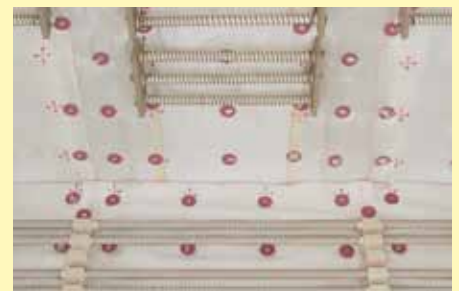
Fabric cover on the fiber roof (and sides) to reduce fiber dust
