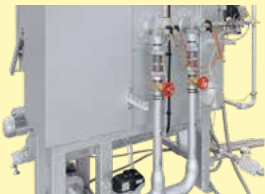
Gas stretch with two burners in the back wall of the furnace
