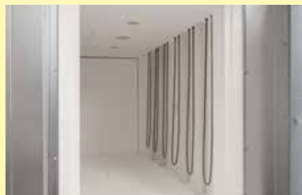
Preheated fresh air blown in via perforated ceramic tubes
