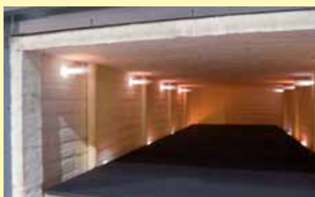
Furnace chamber with eight high-speed burners
