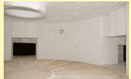
Rotary table with fire-resistant concrete plates to protect the insulation
