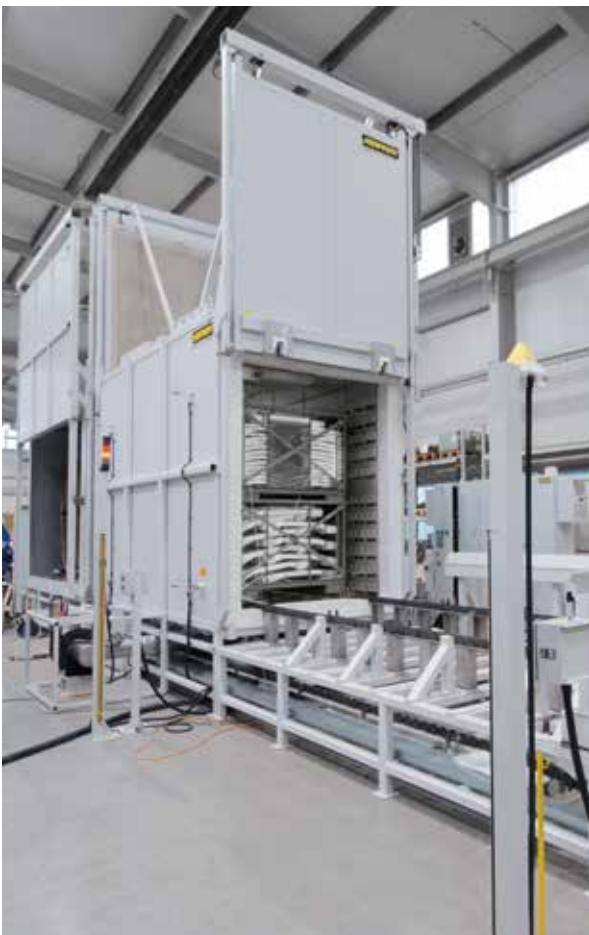
Cycle push-through plant for artificial ageing of aluminum castings
